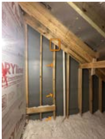
Attic, structural members, twisting & wood splitting
