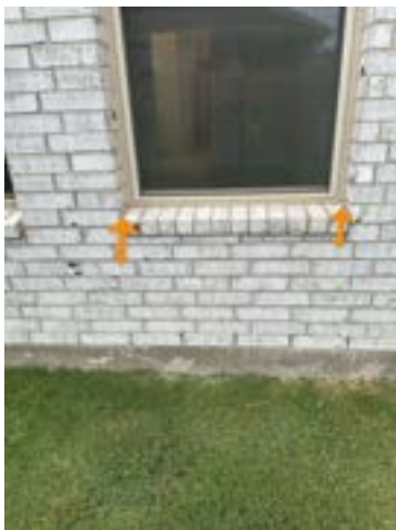
Back of home, windows, caulk/ sealant, deteriorated
