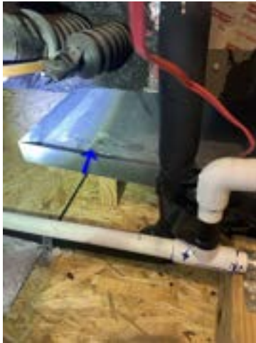
Attic, HVAC unit, drip pan, moisture stains
