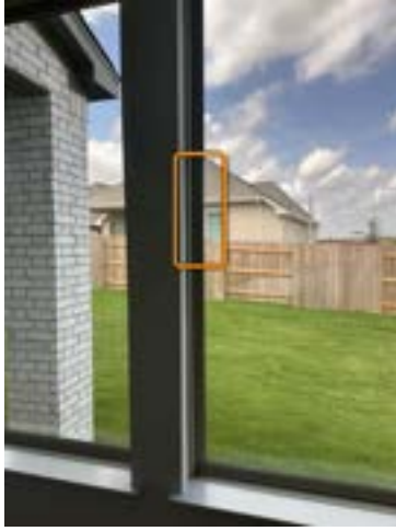
Living room, window, cracked
