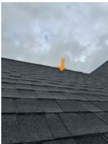
Roof, shingles. loose/ uplifted
