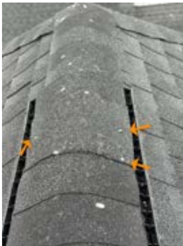
Roof, ridge cap, exposed nails
