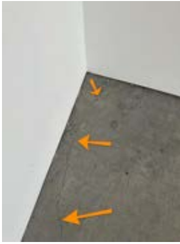
Garage, slab, minor crack
