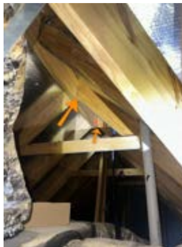
Attic, structural members, separation at connections
