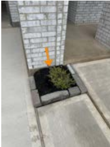
Front of home, foundation, high soil/ mulch
