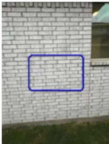
Right of home, brick siding, spalling
