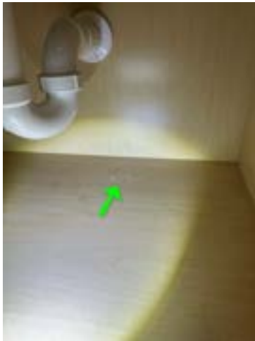
2nd story, sink cabinet, moisture stains, no active leaks
