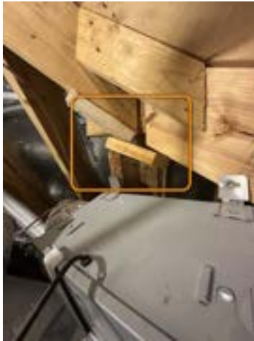
Attic, structural members, separation at connections
