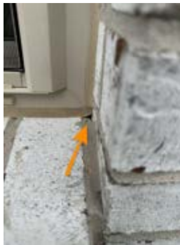
Back of home, windows, caulk/ sealant, deteriorated
