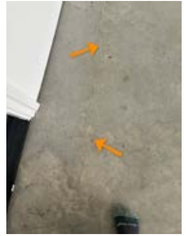
Garage, slab, minor crack
