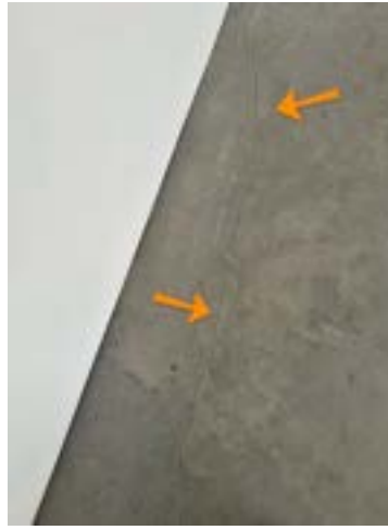
Garage, slab, minor crack
