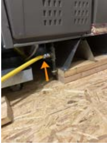
Attic, furnace gas supply, pipe size
