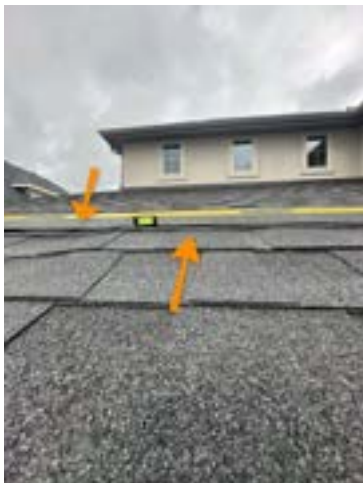
Front of home, roof decking, uneven
