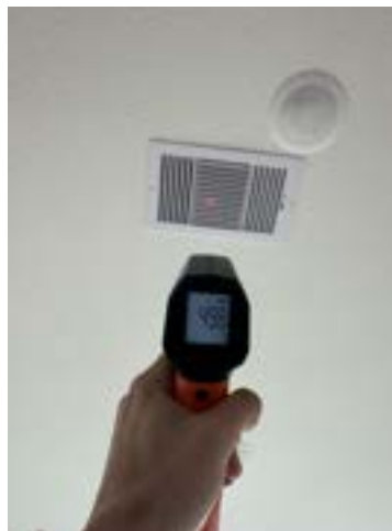
Common area, HVAC supply air vent, temperature reading
