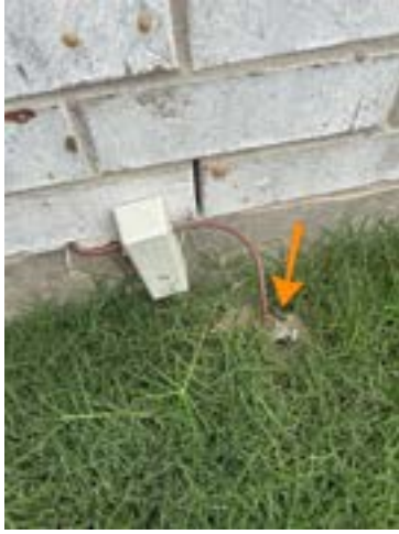
Left of home, grounding rod & wire connection, exposed
