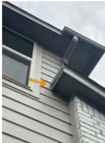
Right side of home, roof to wall connection, insufficient kick out flashing
