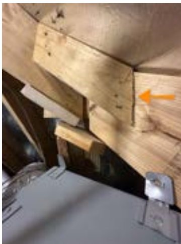
Attic, structural members, separation at connections
