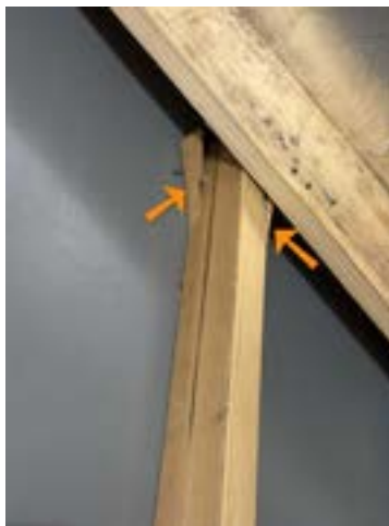
Attic, structural members, twisting & wood splitting
