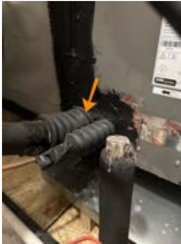
Attic, furnace, flex pipe
