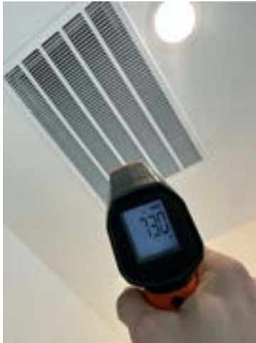
2nd story, HVAC return air vent, temperature reading
