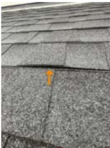
Roof, shingles. loose/ uplifted
