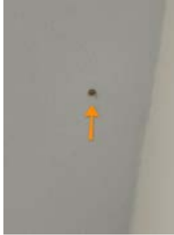
2nd story, bathroom ceiling, nail pop
