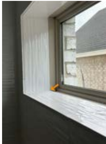
Master bathroom, window above shower, mortar separated
