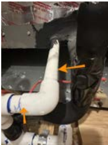
Attic, HVAC unit, condensation
