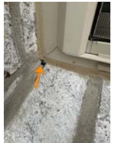
Back of home, windows, caulk/ sealant, deteriorated
