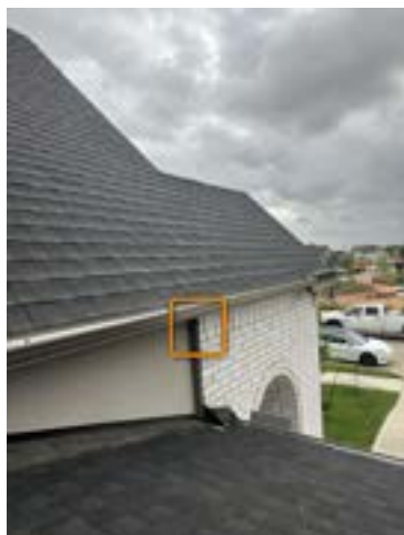
Front of home, fascia board, damaged/ hole
