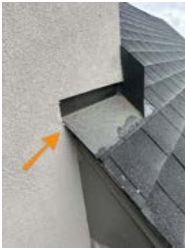
Front of home, roof to wall connection, insufficient kick out flashing
