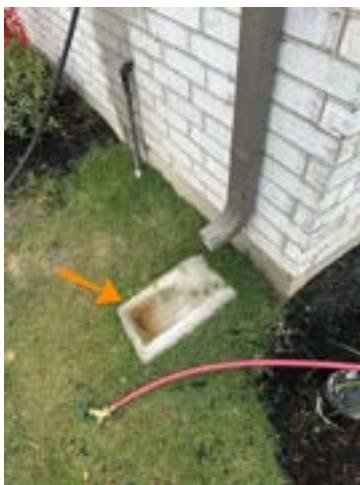
Front of home, splash box, insufficient
