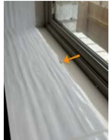
Master bathroom, window above shower, mortar separated
