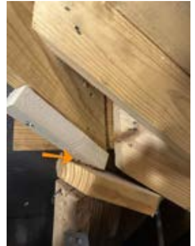
Attic, structural members, separation at connections
