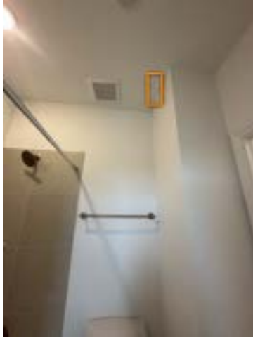
2nd story, bathroom ceiling, nail pop
