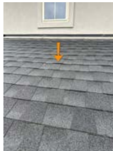
Roof, shingles. loose/ uplifted
