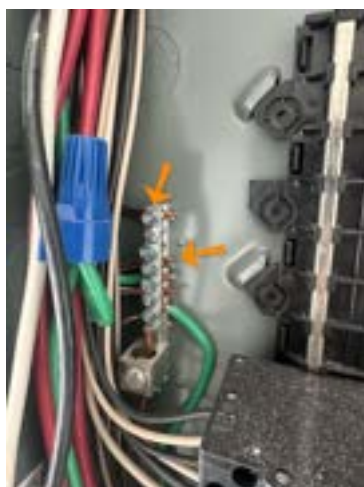
Sub panelboard, neutral bus bar, double tapped
