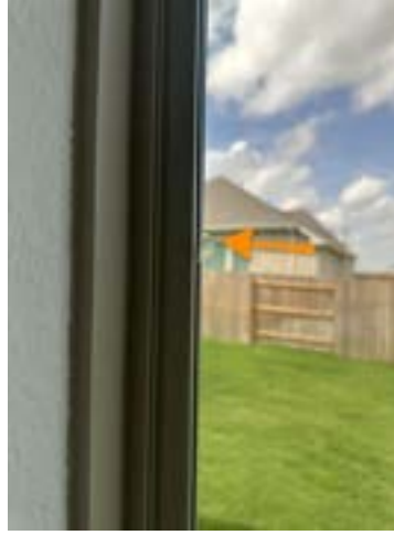
Living room, window, cracked
