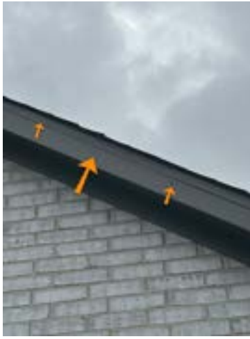
Back of home, fascia boards, nails pops & exposed nails
