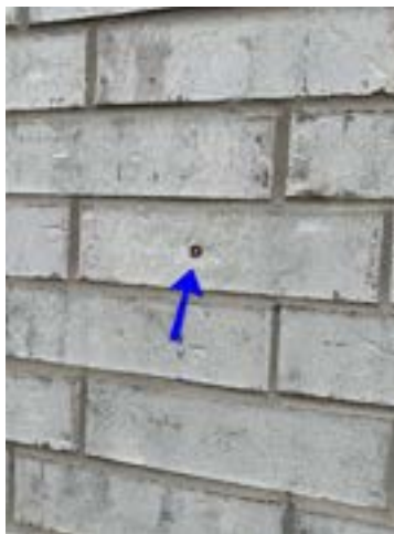
Right of home, brick siding, spalling
