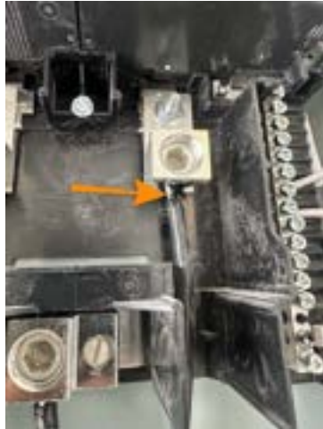
Sub panel, solid aluminum cables, exposed
