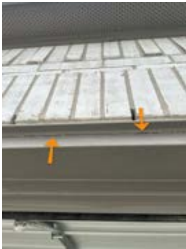
Garage door header trim and lintel, caulk/ sealant separated
