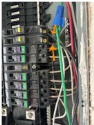
Sub panelboard, circuit breakers, double tapped neutrals
