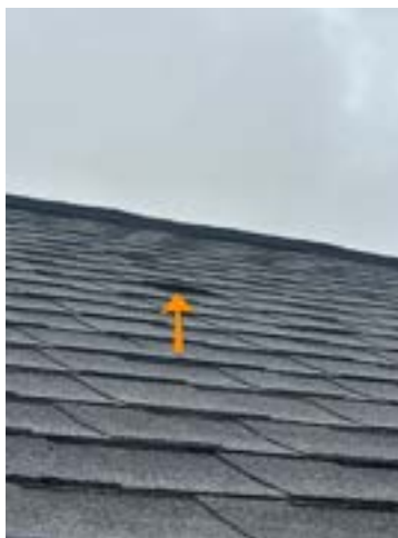
Roof, shingles. loose/ uplifted
