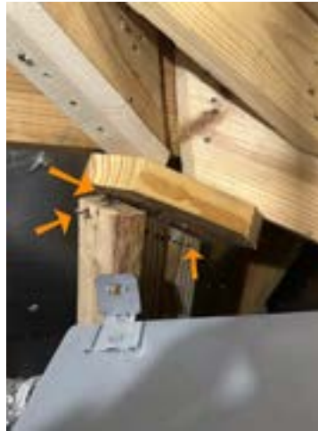
Attic, structural members, separation at connections
