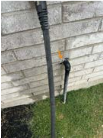
Left of home, electrical conduit, loose
