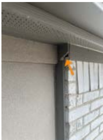
Front of home, fascia board, damaged/ hole
