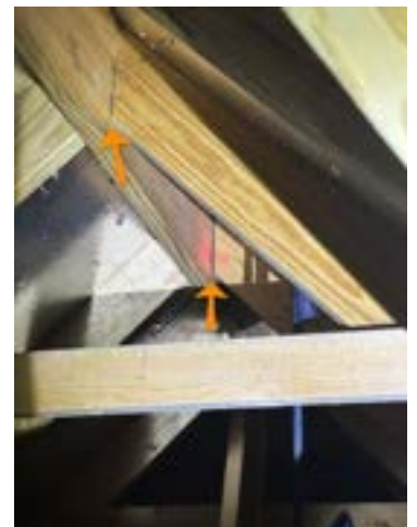
Attic, structural members, separation at connections
