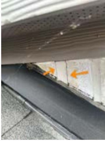
Back of home, brick siding, mortar joint cracked
