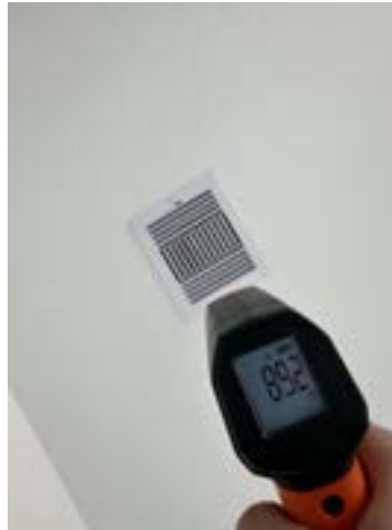
2nd story, HVAC supply air vent, temperature reading
