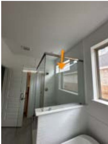
Master bathroom, window above shower, mortar separated
