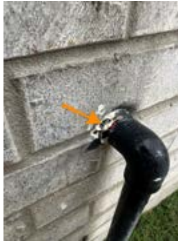
Left of home, electrical conduit, loose
