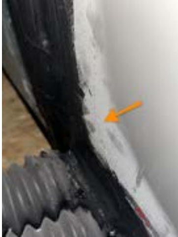
Attic, HVAC unit, condensation
